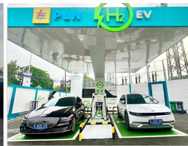
Green Hydrogen EV Car Charging Station
